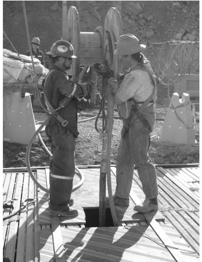
Figure 13. Miners cinching bolts coupling wire rope lanyard to pump hose and crane hoist rope.
